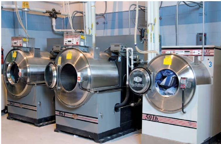
While the new tunnel was being installed, CDHL worked overtime to process incoming linen using three washer-extractors originally installed with the 1992 tunnel system. Installation was planned for the time its hospital customers had their lowest linen usage of the year.
