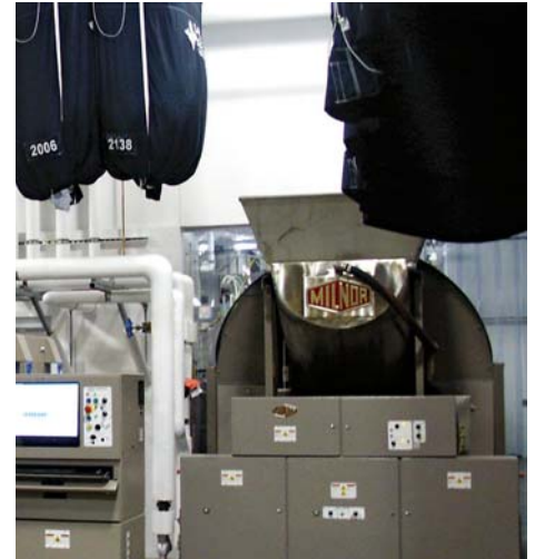
Two eight-module tunnel washers anchor the plant. HSHS is using only one until other hospital customers are brought into the fold.
